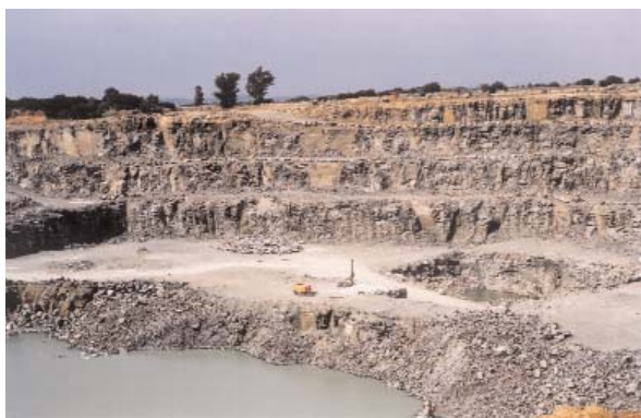
Percussion drilling in preparation for blasting fresh dolerite for aggregate at the Olive Hill Quarry northeast of Bloemfontein.
