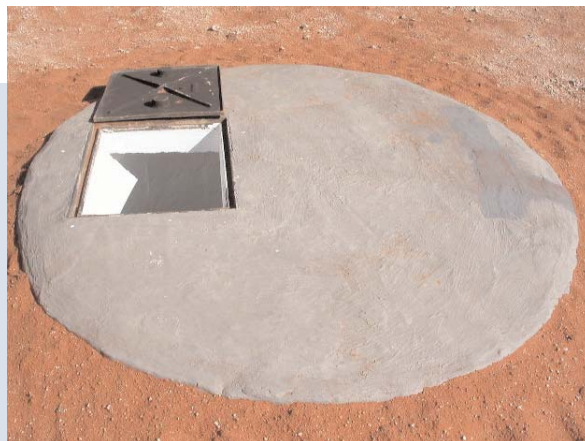
Photographs of some of the upgraded vaults that have been constructed: (1) the new and old vaults of the Upington station, (2) inside the new vault of the Calvinia station, (3) the new vault of the Lephalale station, (4) the new vault of the Prieska station, and (5) the new vault of the Upington station. Note the distinct improvement between the old and new vaults.
